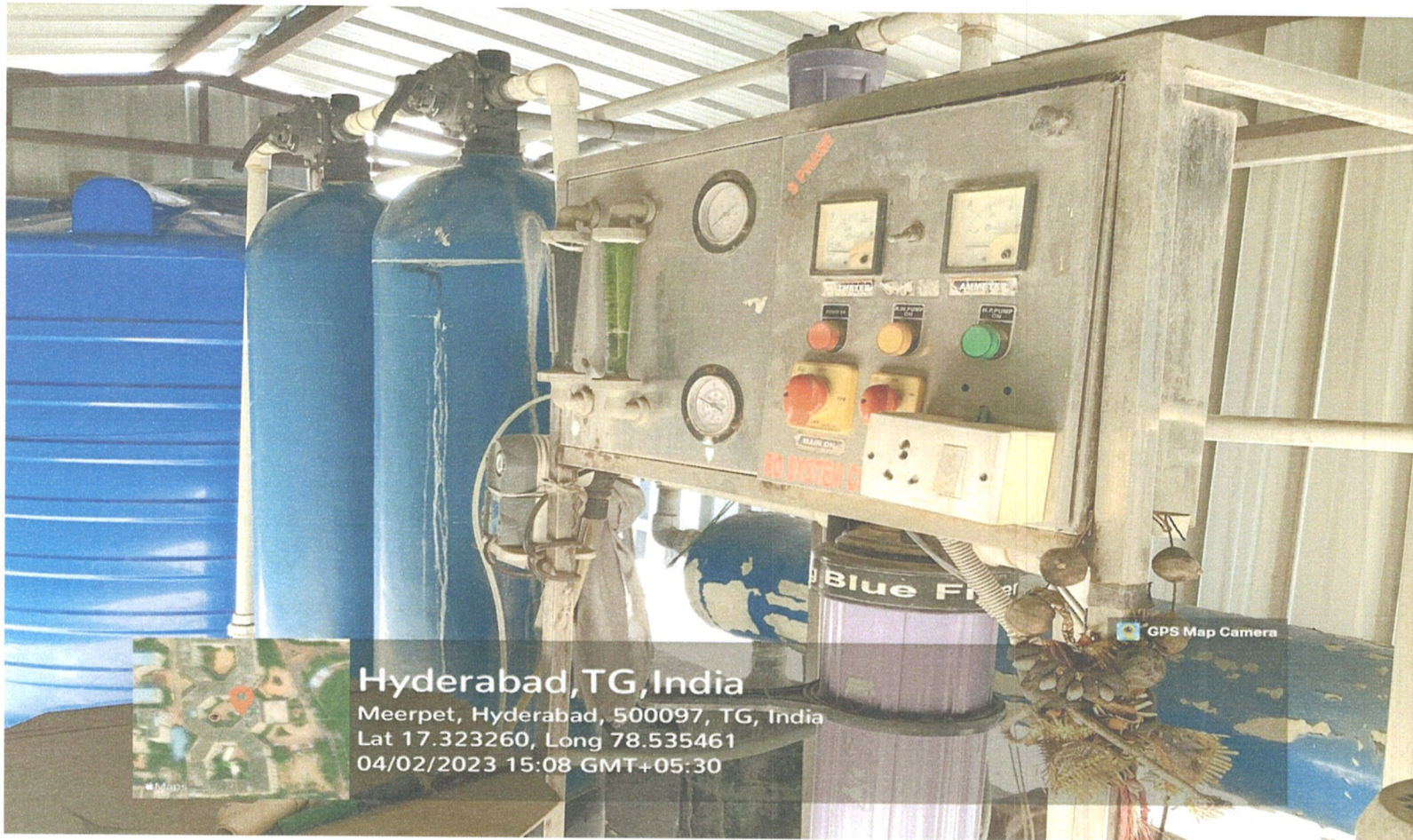
RO Water Filter System
