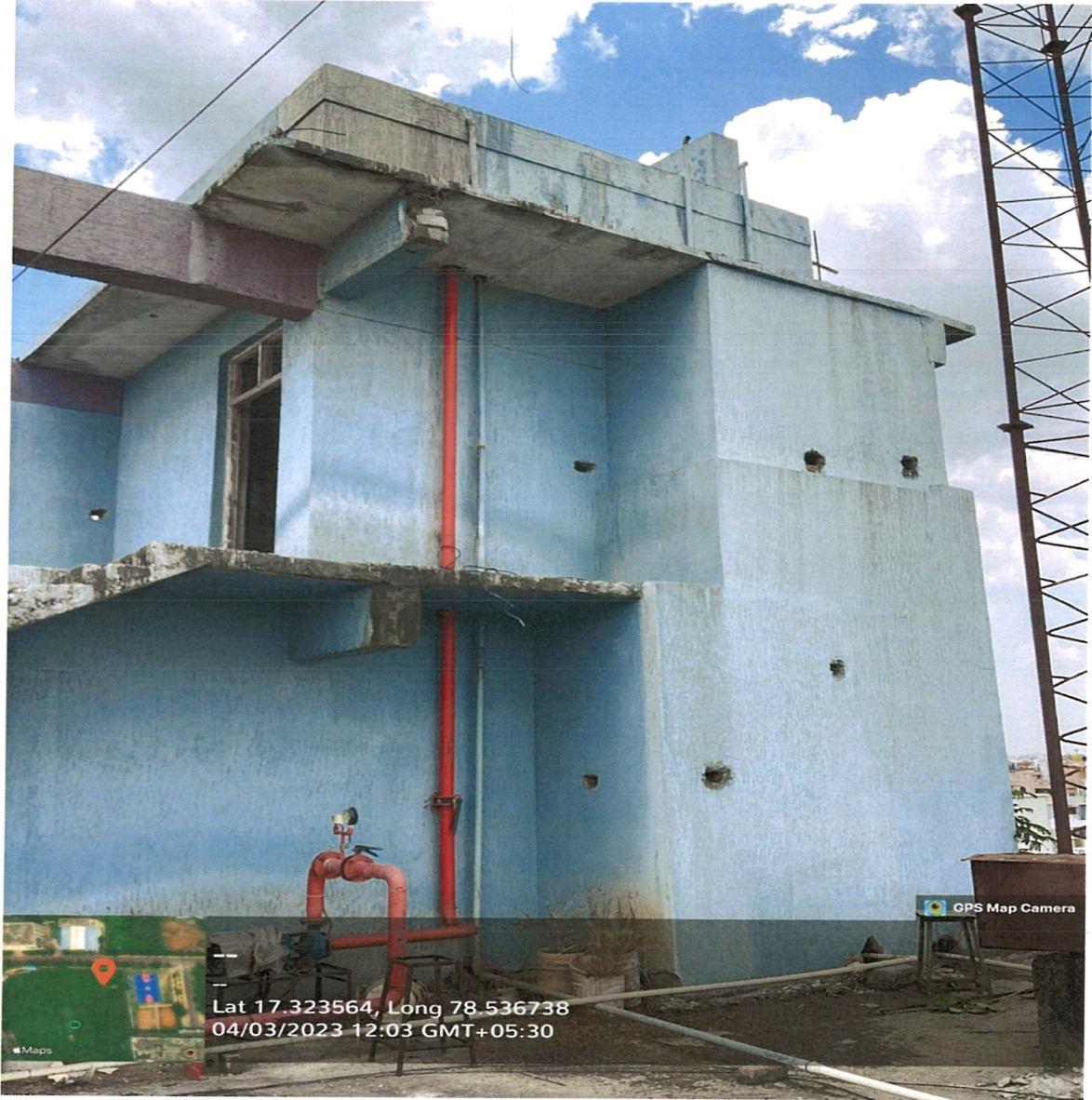
Water Tank for Distributing Water in the campus
