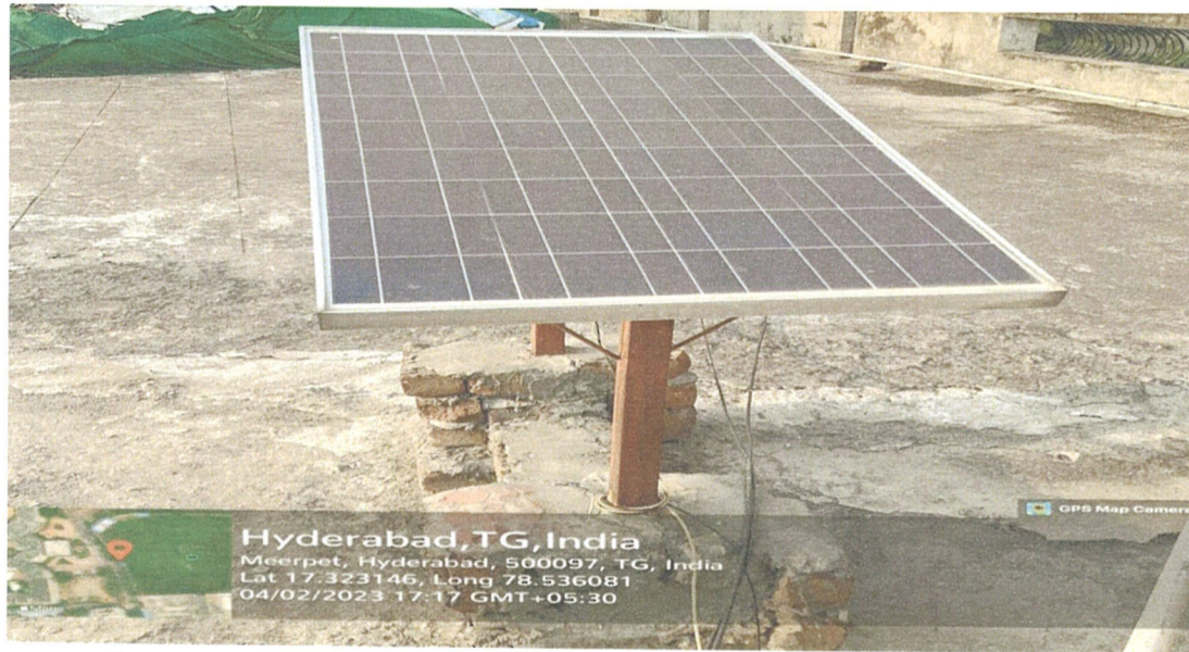
Solar Panels for Electrical Engineering Electronics engineering lab Electrification to save Energy
