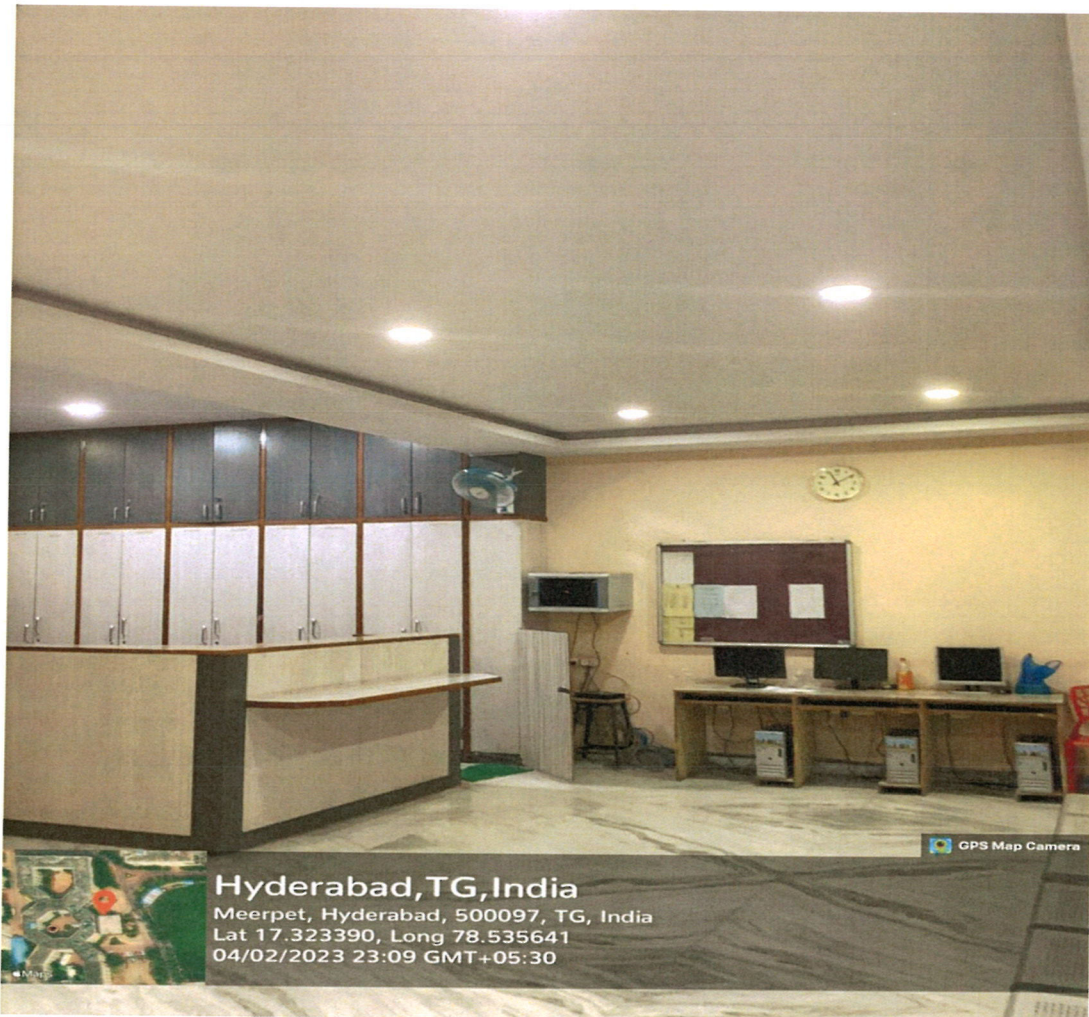
LED Bulbs Installed within the Campus for Energy Conservation
