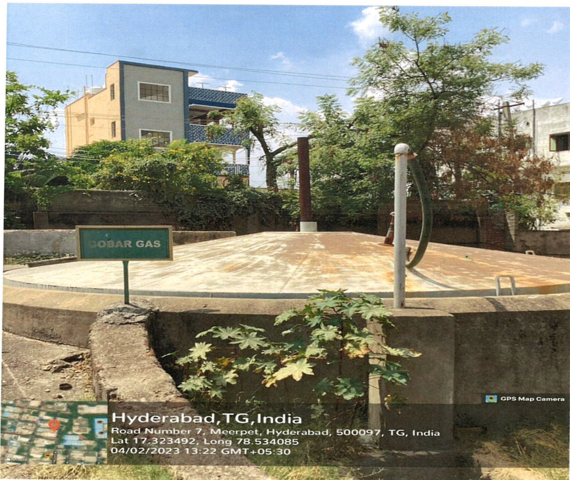
Biogas Plant Unit
