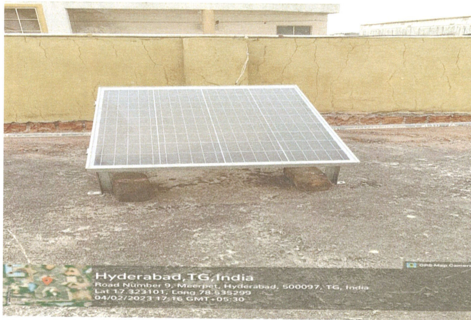
Solar Panels for Electrical Electronics Engineering lab. Electrification to save Energy
