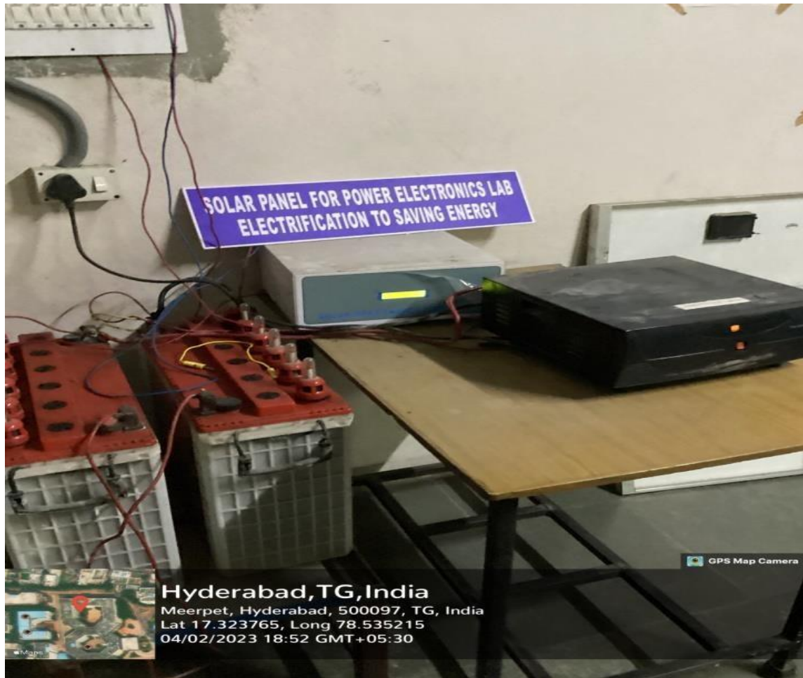
Solar Power for Power Electronics Lab for Energy Conservation
