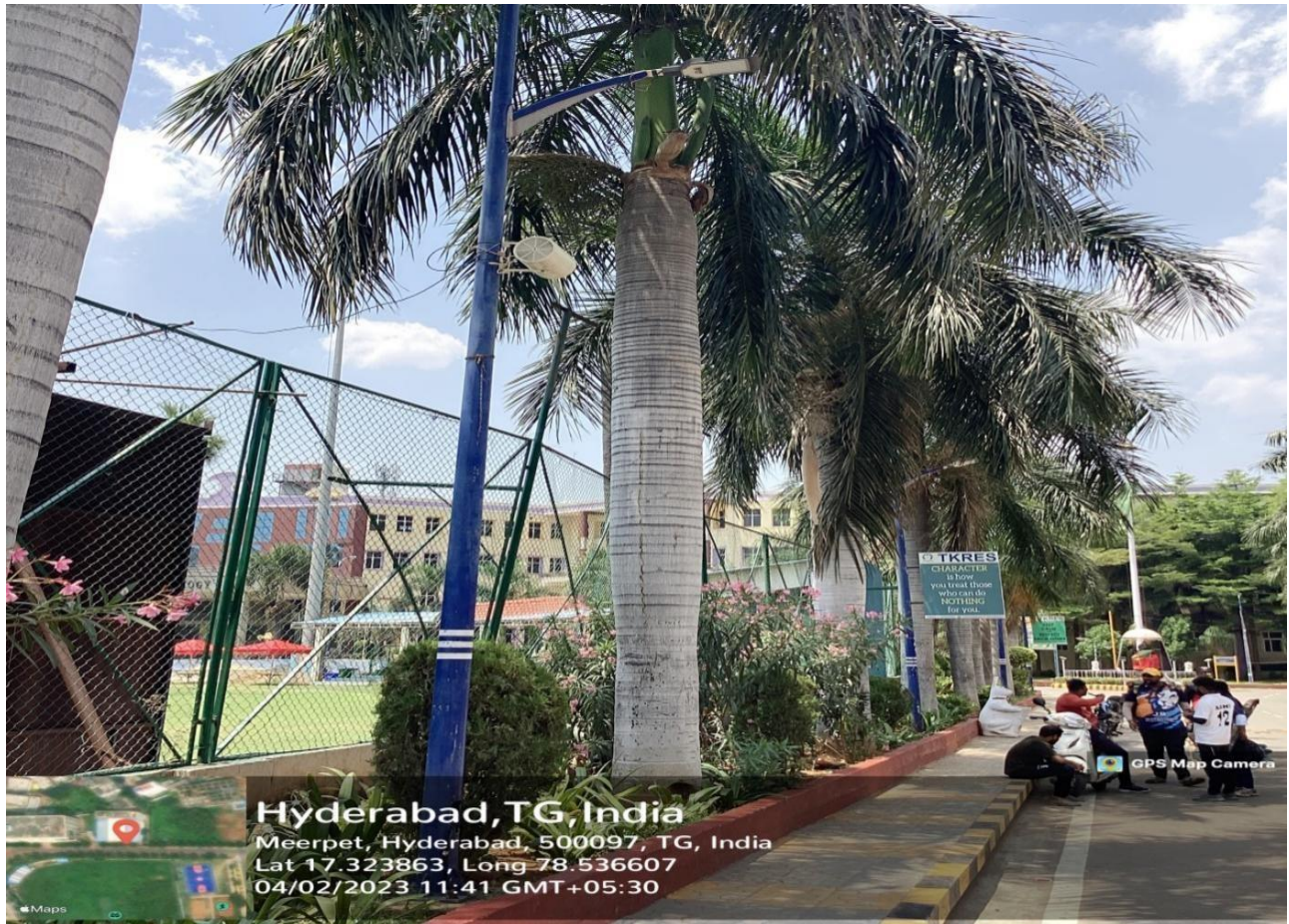
Sensor Based Street Lights for Power Conservation
