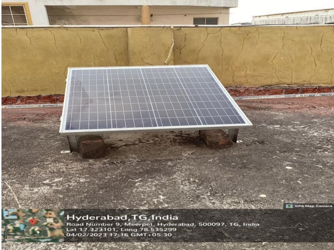
Solar Panels for Electronics Lab Electrification to Save Energy
